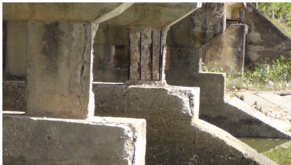
Figure 3-18. Corrosion recorded at Ho Phong sluice gate
